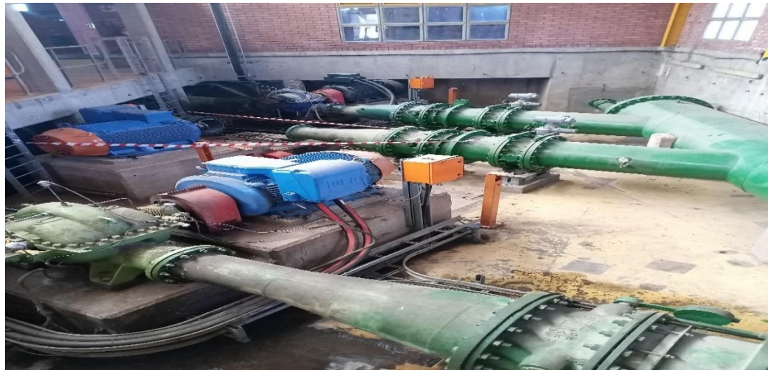
Figure 5: The photo depicts infrastructure pumps abstracting raw water from Leeuwkraal Dam to Temba WTW plant for purification and distribution to the community at the time of inspection.
