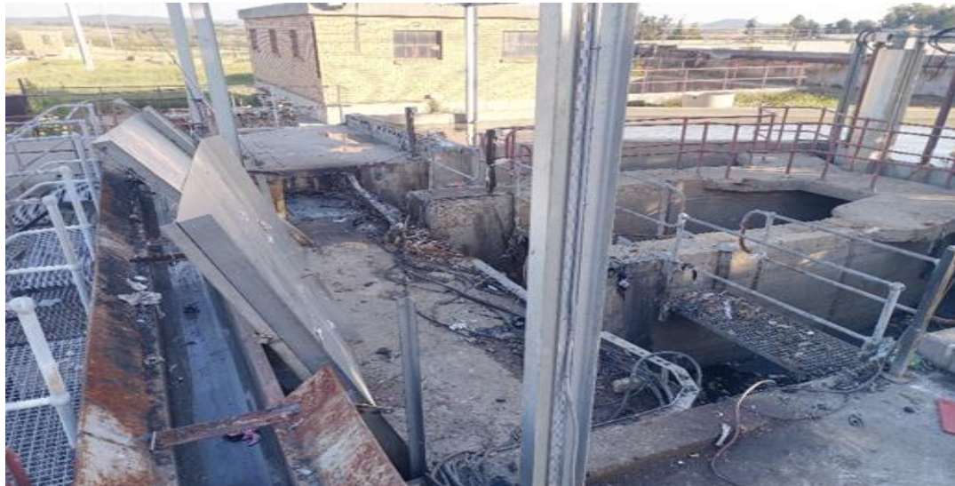
Figure 2: The photo depicts, amongst other things, a conveyer-belt which was not working due to faulty automated mechanical screens/bars having been removed for repairs at the inlet area, Rooiwal WWTW at the time of inspection.
